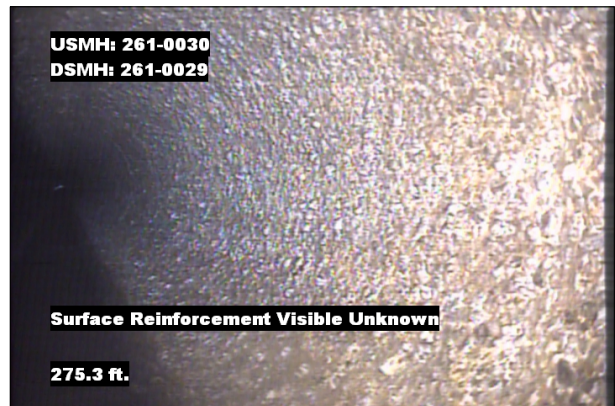
Photo: 261-0030_261-0029_SRVZ_275.3.jpg, VCR No.: 1 275.3FT, Surface Reinforcement Visible Unknown, from 09 to 03 o'clock, within 8 inches: NO
