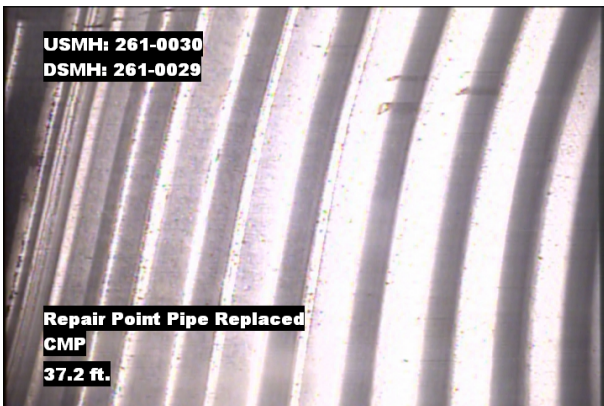
Photo: 261-0030_261-0029_RPR_37.2.jpg, VCR No.: 1 37.2FT, Repair Pipe Replaced, within 8 inches: YES, REMARK: CMP
