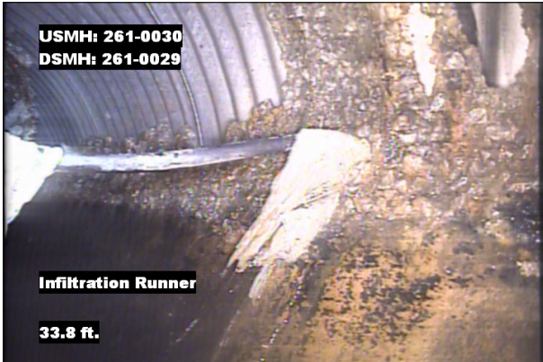
Photo: 261-0030_261-0029_IR_33.8.jpg, VCR No.: 1 33.8FT, Infiltration Runner, at 02 o'clock, within 8 inches: YES
