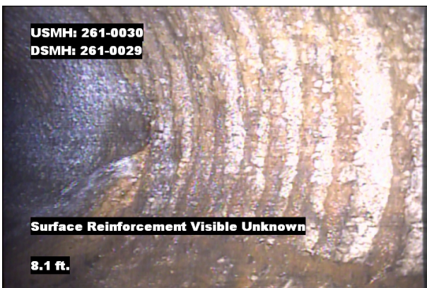
Photo: 261-0030_261-0029_SRVZ_8.1.jpg, VCR No.: 1 8.1FT, Surface Reinforcement Visible Unknown, from 09 to 03 o'clock, within 8 inches: YES
