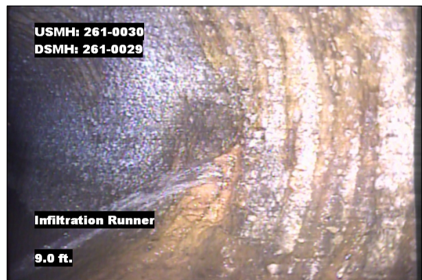
Photo: 261-0030_261-0029_IR_9.0.jpg, VCR No.: 1 9FT, Infiltration Runner, at 02 o'clock, within 8 inches: YES
