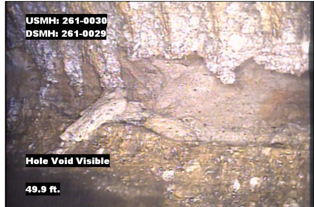
Photo: 261-0030_261-0029_HVV_49.9.jpg, VCR No.: 1 49.9FT, Hole Void Visible, , at 02 o'clock, within 8 inches: NO
