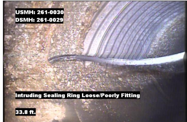
Photo: 261-0030_261-0029_ISSRL_33.8.jpg, VCR No.: 1 33.8FT, Intruding Sealing Ring Loose/Poorly Fitting, 5% of cross sectional area, from 10 to 02 o'clock
