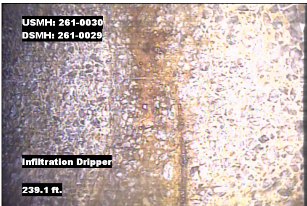
Photo: 261-0030_261-0029_ID_239.1.jpg, VCR No.: 1 239.1FT, Infiltration Dripper, at 12 o'clock, within 8 inches: YES
