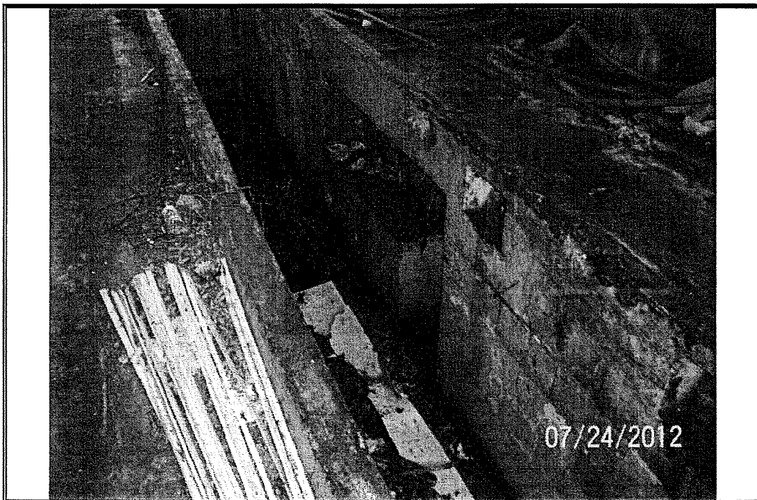
Photo # 6: View of the yellow paint identified as containing lead at 1.36 %.
