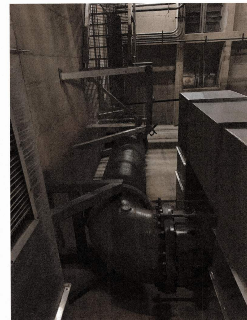
FORCE MAIN DISCHARGE - NORTH VIEW
