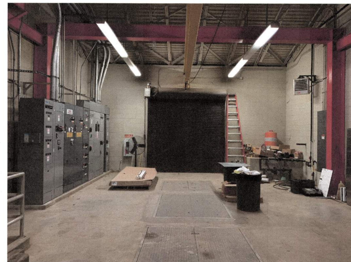
ELECTRICAL ROOM - NORTH VIEW
