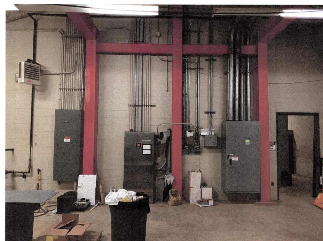
ELECTRICAL ROOM - EAST VIEW
