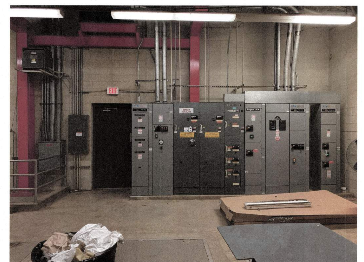
ELECTRICAL ROOM - WEST VIEW
