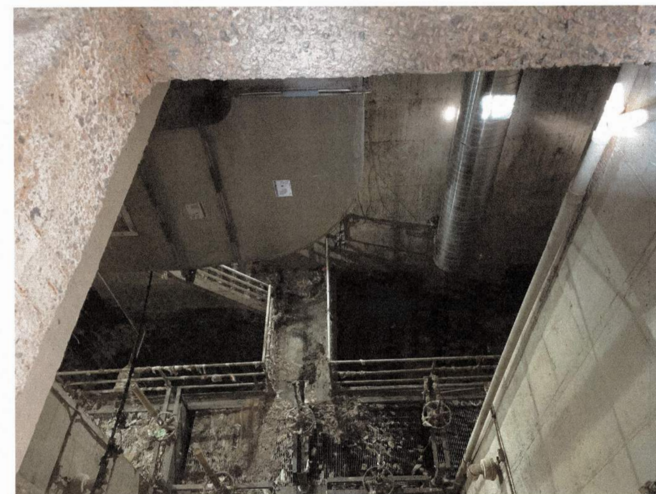
WET WELL - WEST END
