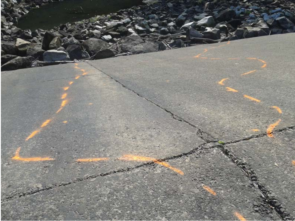
Figure 4: View the northeast anomalous area on the downstream face of the dam.
