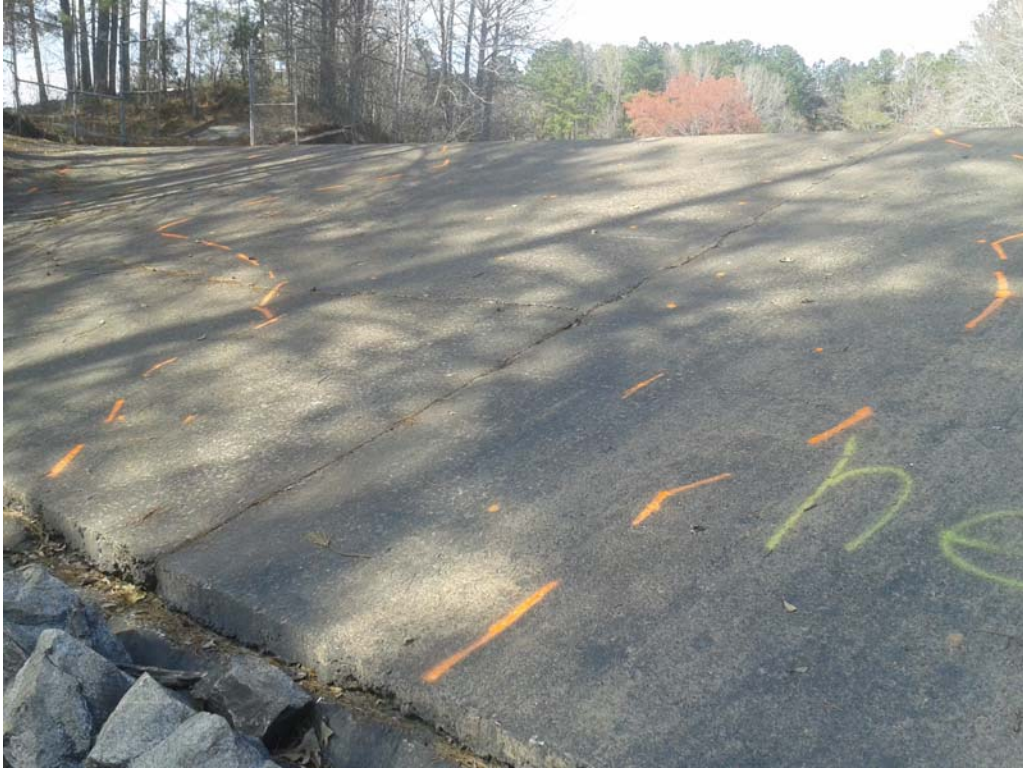
Figure 6: View the northwest anomalous area on the downstream face of the dam.
