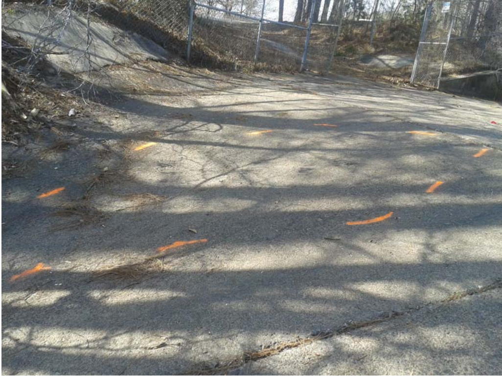
Figure 8: View the possibly anomalous area in the northwest corner of the dam.
