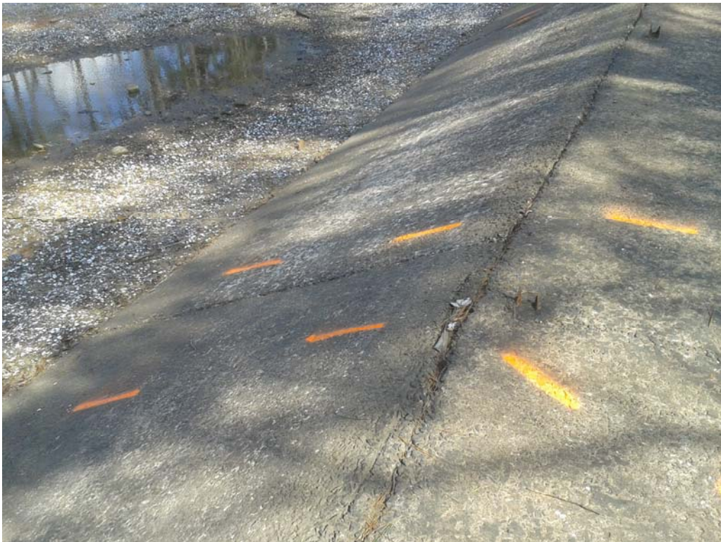
Figure 3: View of one of the anomalous areas on the lakeside of the dam.
