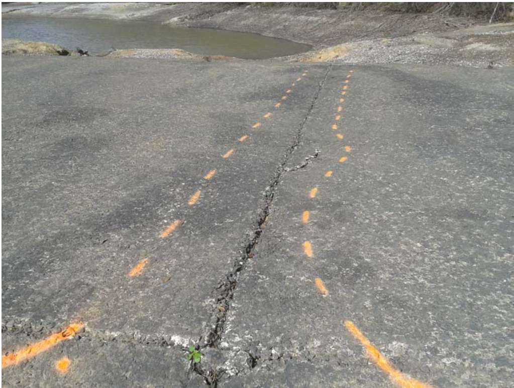
Figure 5: View the anomalous area to the northeast along the top of the dam.
