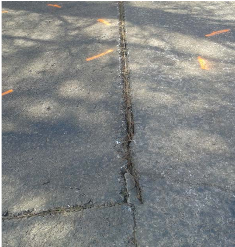
Figure 9: View the damaged control joint at the northwest end of the dam between the top and the downstream face of the dam.
