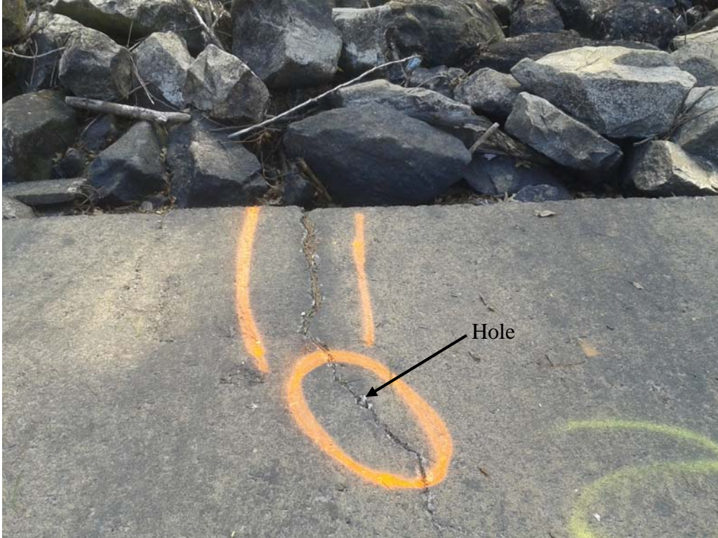
Figure 2: View of the hole found along a crack on the downstream face of the dam.
