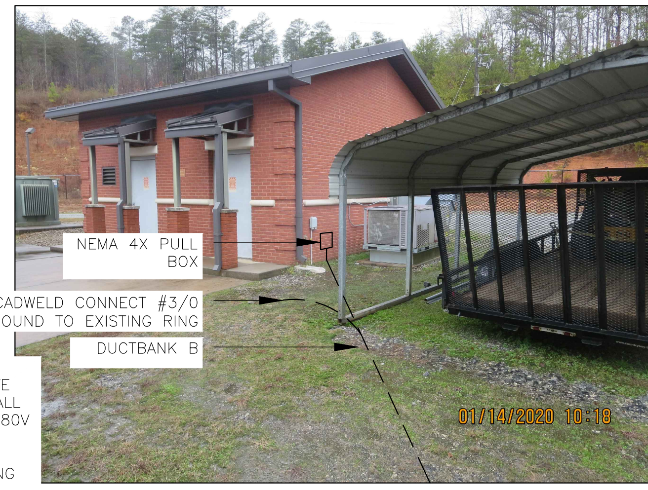
FIGURE 2: EXISTING ELECTRICAL ROOM
