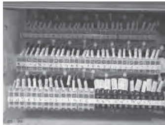
Master Terminal Blocks at Bottom (Class C Wiring)
