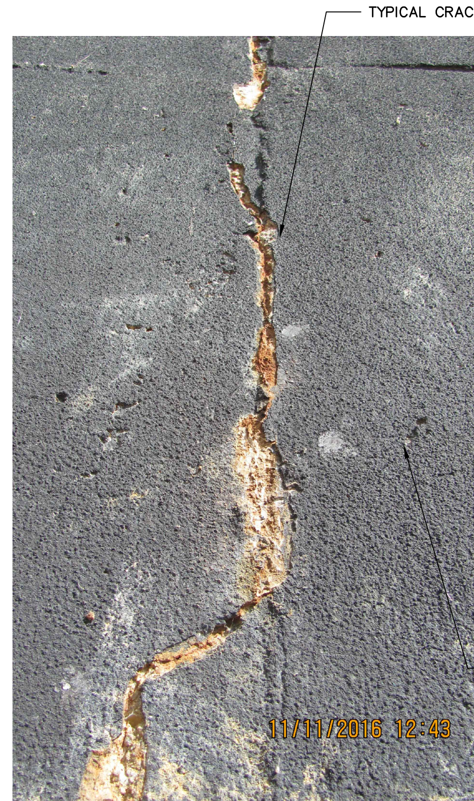
PHOTO 2: TYPICAL CRACK AT JOINTS
