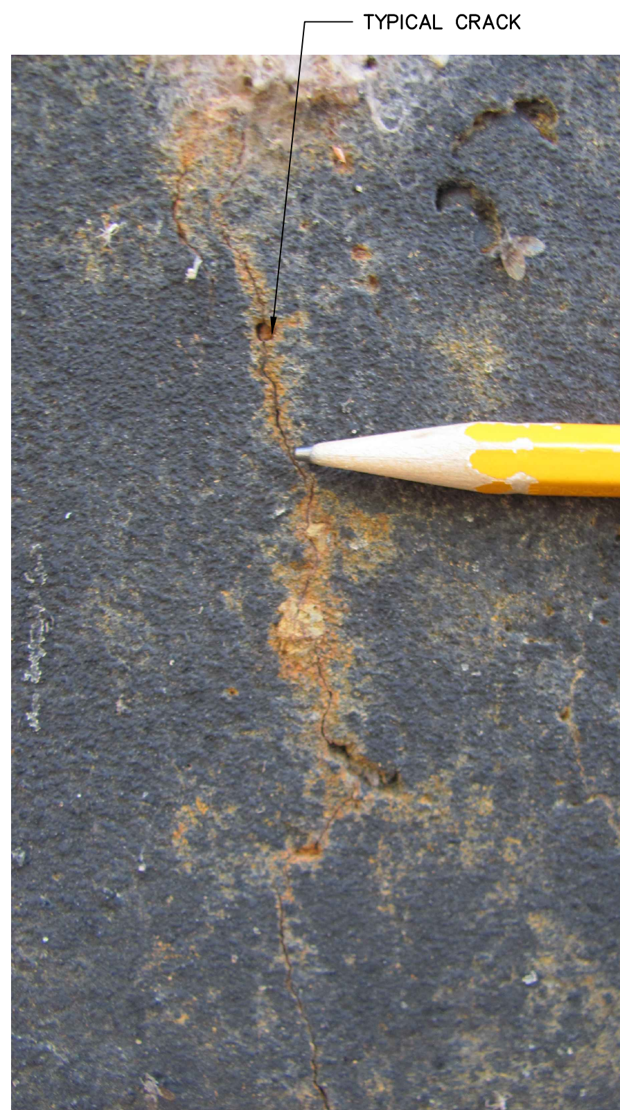
PHOTO 1: TYPICAL INTERIOR WALL CRACK
