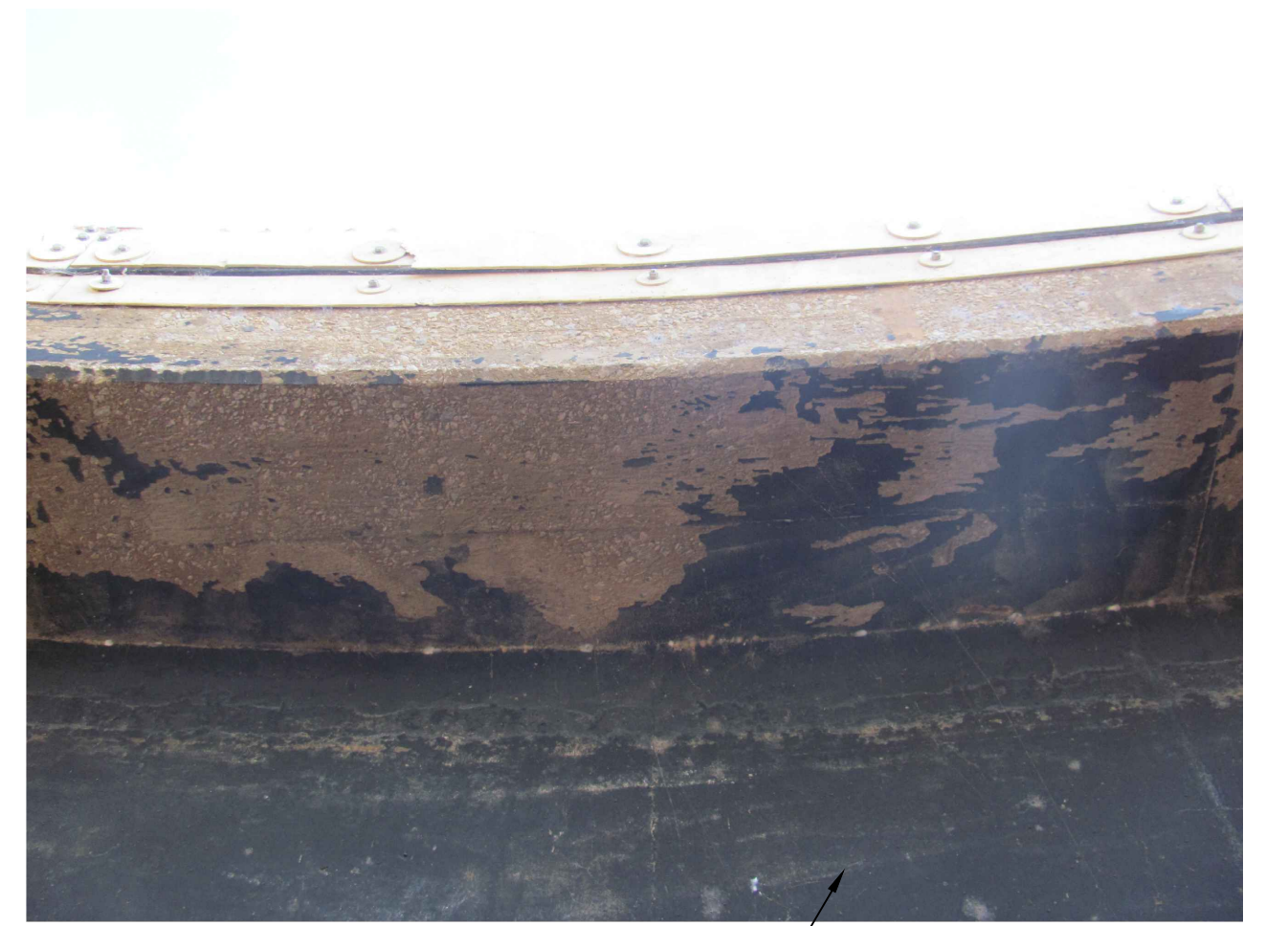
PHOTO 5: TYPICAL COATING FAILURE
